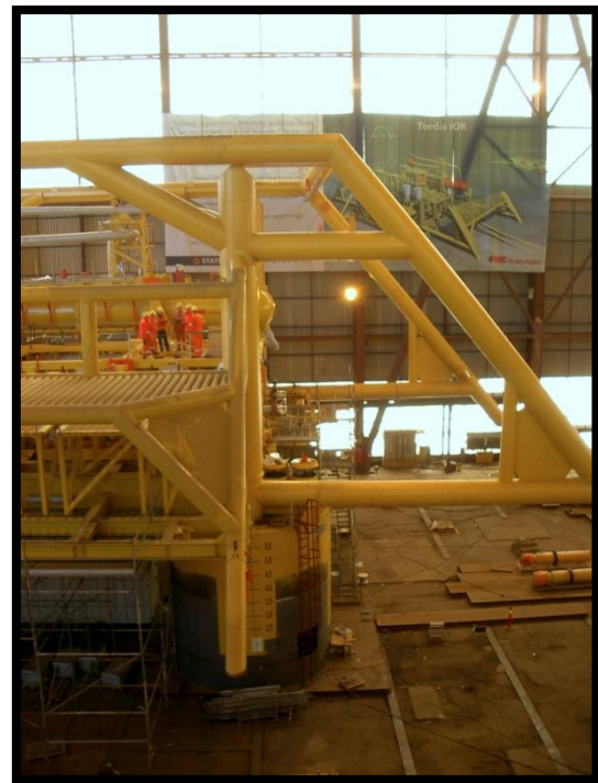
THE FIRST FULL SCALE UNDERWATER SEPARATION MODULE UNDER CONSTRUCTION AT GRENLAND GROUP
